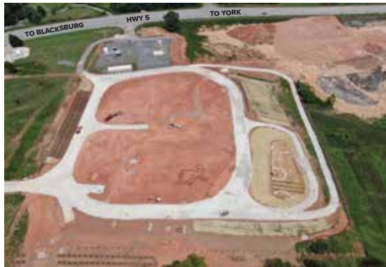
Civil site work is currently underway with facility construction planned to begin in August. Completion is slated for spring of 2023.
