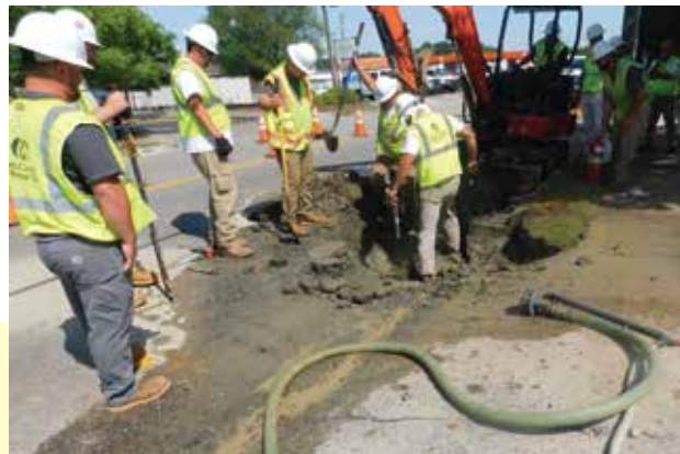
Crews repair a damaged pipe on Camden Avenue. In his role as Hometown Security Coordinator, Glenn responds to incidents within the city to ensure the safety of the area, provide resources if needed and mitigate the impact on neighborhoods and area businesses.
